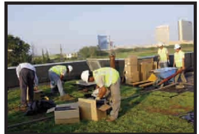
Employees of Plant Connection and Steven Dubner Landscaping install the green roof system as a demonstration project.
